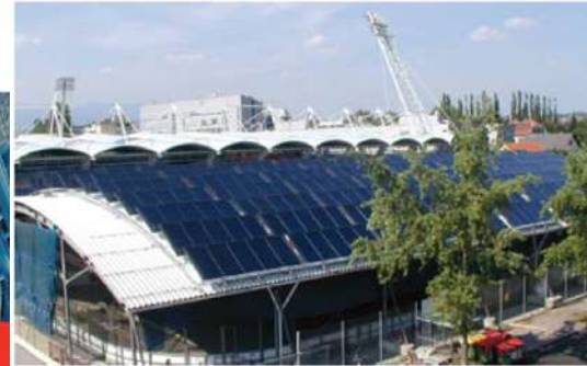
Figure 23: Solar district heating plant in Graz, AT.
