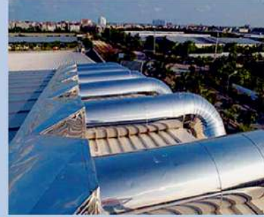
Figure 2: Solar air heating system in textile industry in Vietnam
